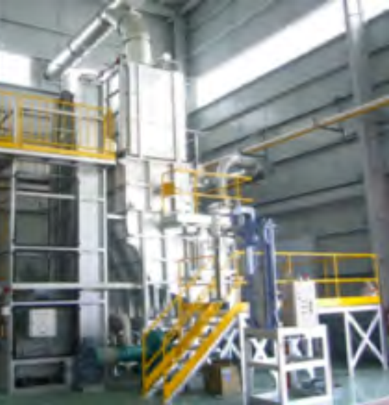
Tower or Stack Melter
